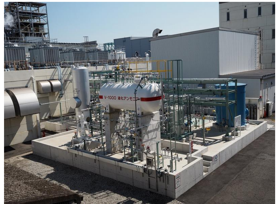
Ammonia supply unit
