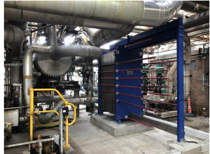
Figure: Example of standard decarbonisation project. Install improved heat exchanger to reduce steam, and hence fuel consumption (~10kt/y CO 2 )
