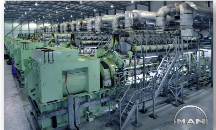
20MW each – V18 MAN (fuel oil engines)
