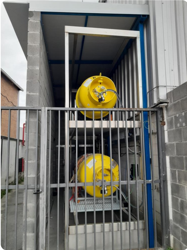
2x 500 kg Ammonia tanks at H2SITE's site
