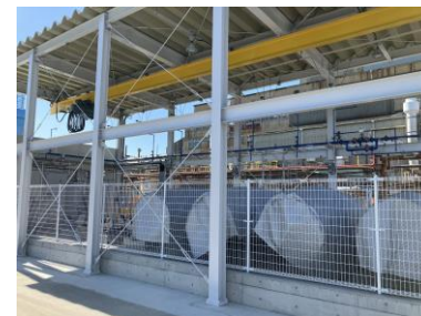
Storage tank for ammonia fuel
