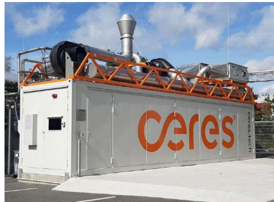
MW-class SOEC system installed at test site in Germany
