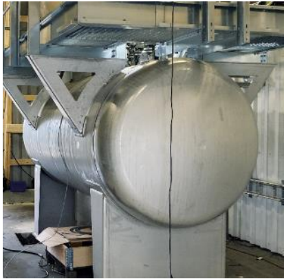
Ammonia service tank
