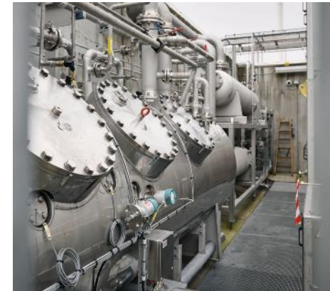
Ammonia catch system
